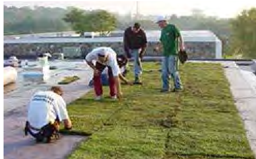
This photo shows the installation of a green roof which can reduce indoor temperatures and manage rainwater runoff.
